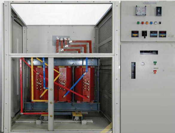
Compact Sub-station with Dry Transformer
